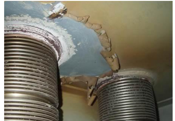
External Penetration Hot Spot
